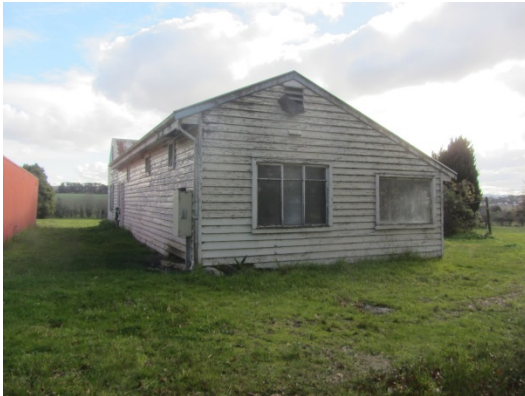
Figure 6. East view of bedroom wing, showing gable end of dining - kitchen wing (Source: Context 2017)
