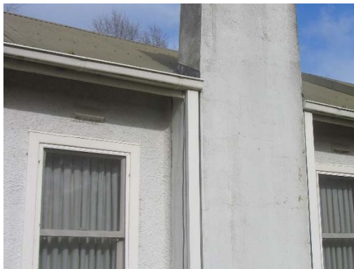
Figure 9. Chimney with smooth finish contrasted with the rough cast Conite walls (Source: Context 2017)
